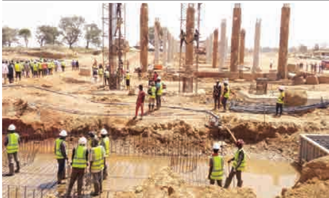
Workers at the construction site of the ongoing Kaduna-Eastern Bye-Pass Project, in Kaduna State yesterday.
